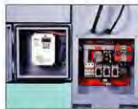
▲ Electrical box & inverter
